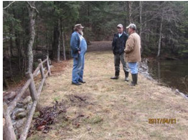
6. Top of dam right – Settlement
