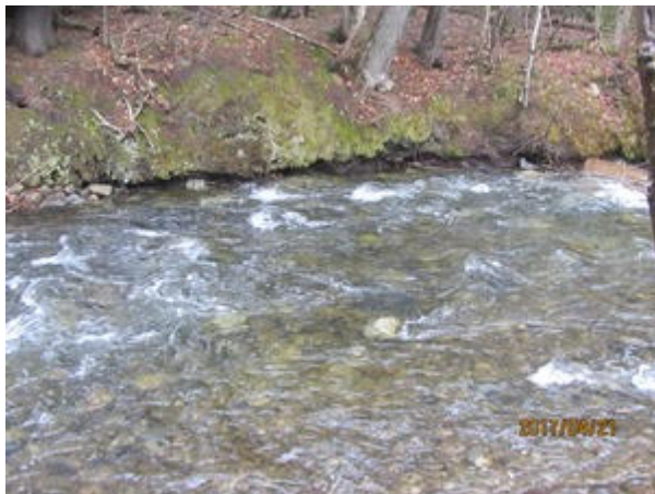
3. Channel erosion undercutting left abutment
