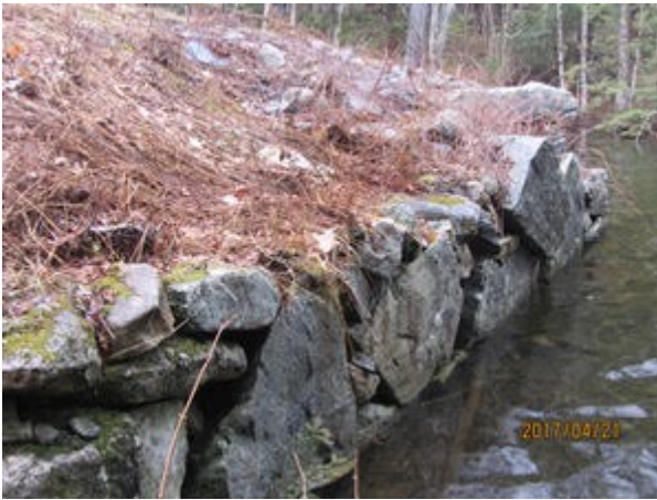
11. Toe right. Stone displacement
